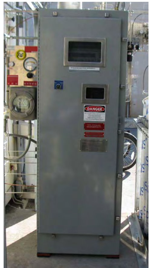
TAI Model 6400E-TSG installed on a California Refinery Steam Methane Reformer
