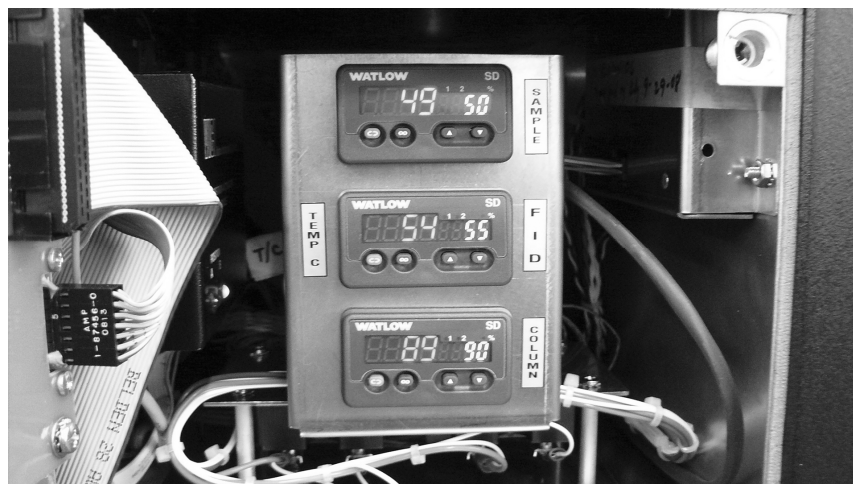
Figure 2-1: Internal Temperature Controllers
